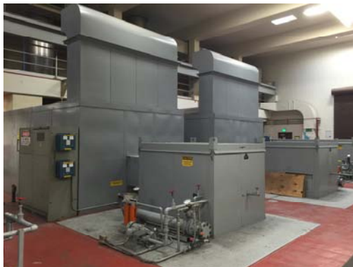
Diesel Engine Enclosures at OLEPS
