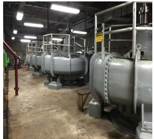
OLEPS Pump Room
