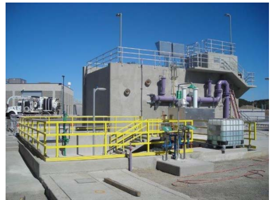
Filter Feed Pump Station and Tertiary Filter
