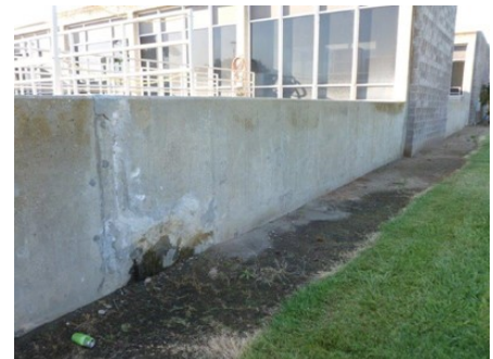
This water basin has a leaking crack in the concrete.
