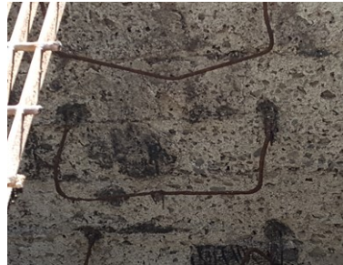
This ladder (yes, that's a ladder) needs replacement.
