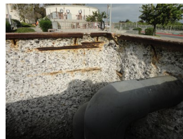
Biogenic sulfide corrosion had severely damaged this influent splitter box.
