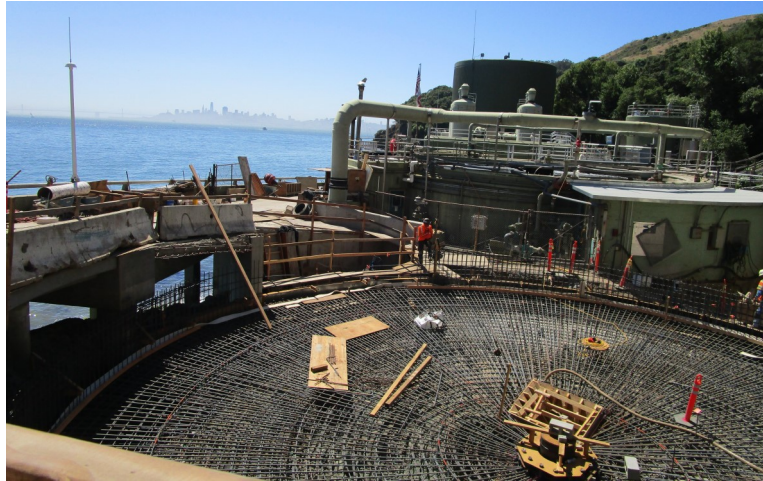
Primary Clarifier Designed by TJCAA—Currently under Construction in the San Francisco Bay Area
