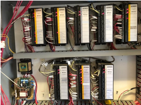
Genius Series I/O Installed in the 1990s Photo - Michael Eriwin
