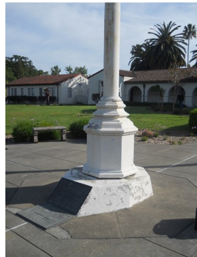
Flagpole Base Before Corrosion Prevention Measures Photo - J. Darby Howard
