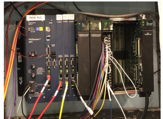
This GE PLC is an obsolete RX7i that was an upgrade to a long-obsolete 90-70.
