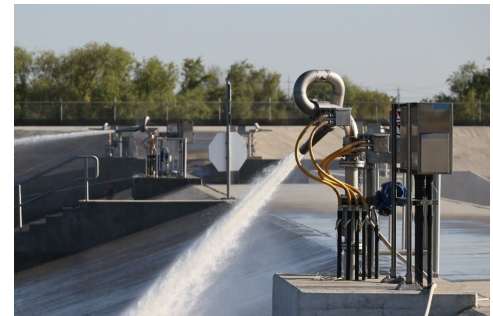
Basin Wash Water Applied by a Remote-Controlled Monitor
