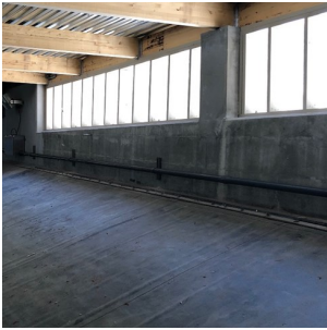
Post-construction testing verified that the reservoir interior was free from contaminants and ready to go back into operation.
